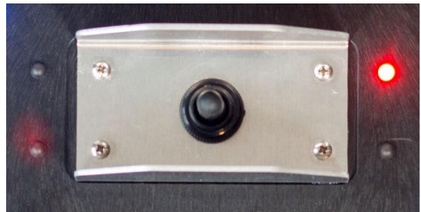
With the switch set to the centre, red-red position the A side lights are blank indicating solid amber.
