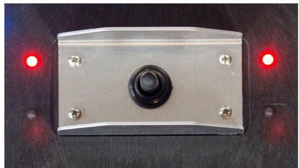
Once the amber time has completed the controller and light will display red-red.
